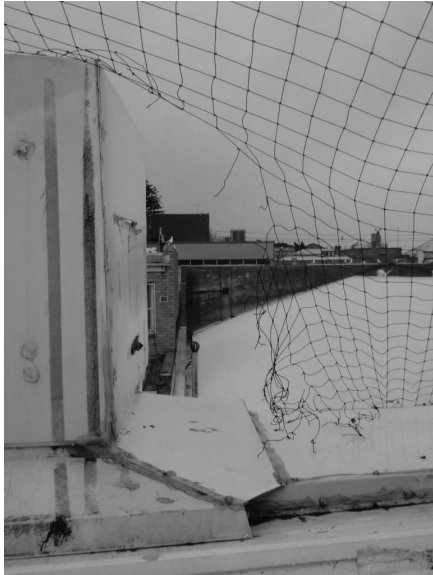
Example of poorly maintained rooftop netting system – holes allow gulls in but they can't always find their way out – Frankston CAD 2011
