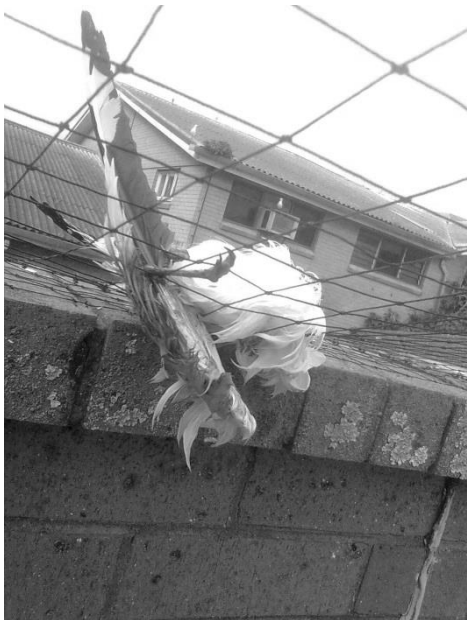
Dead gull trapped in netting at roof edge – Frankston CAD 2012
